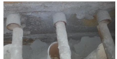
Corroded/damage blowpipe connector
